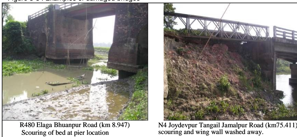
Figure 3-3 : Examples of damaged bridges
