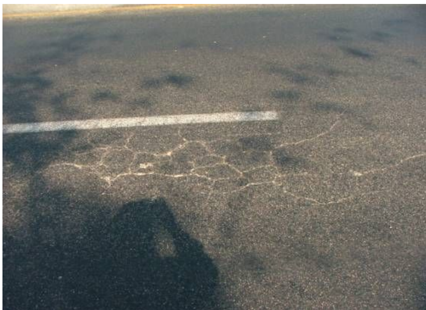
Figure 3-9 : Top Down Cracks, N1 Dhaka-Chittagong
